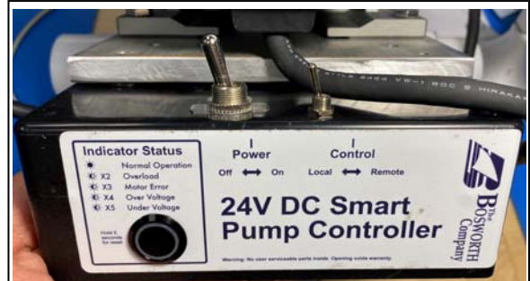
Pump Control box showing manual and remote activation switches on top of box and fault status indicator on side Figure 6
