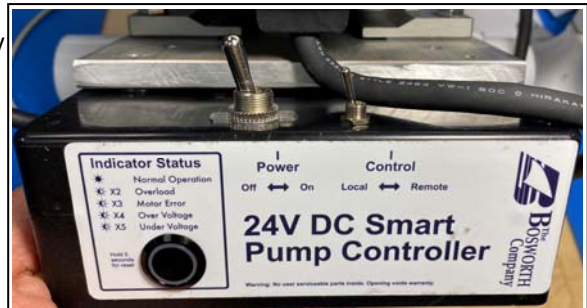
Pump Control box showing manual and remote activation switches and fault status indicator Figure 8
