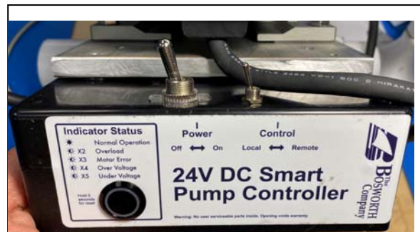
Pump Control box showing manual and remote activation switches and fault status indicator Figure 7
